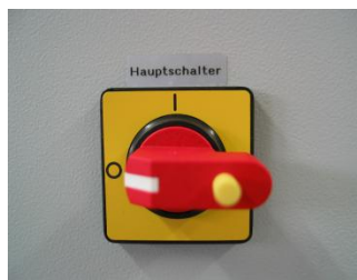
Figure main switch on the front panel door (at large Chillers)
