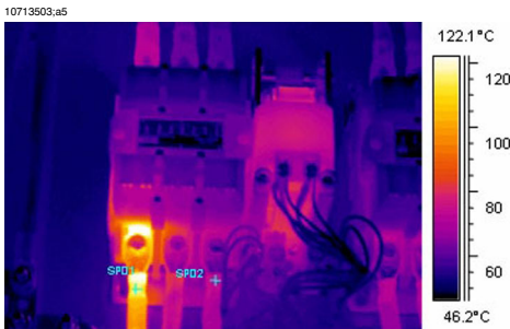
Figure 17.9 An infrared image of indoor electrical equipment (2).
