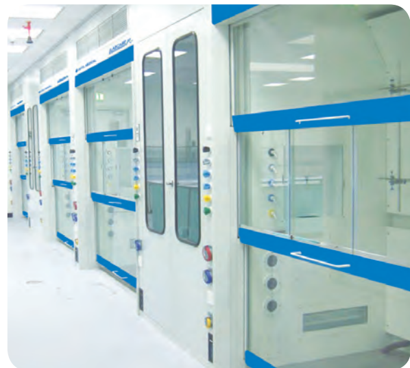
Walk in Fume Cupboard
